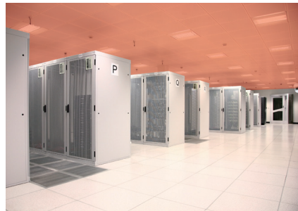
Ceiling protection at Data center
